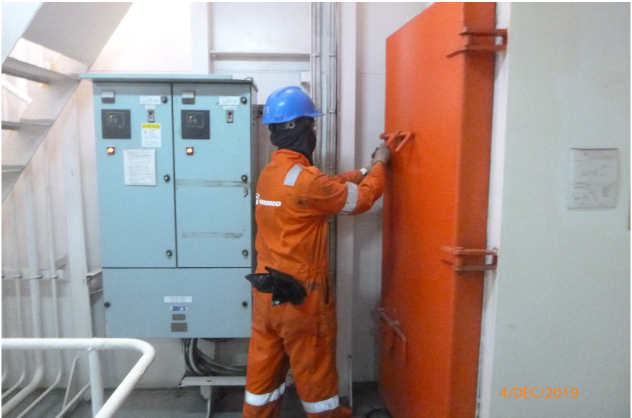
ENGINE ROOM DOORS LOCKED DOWN
